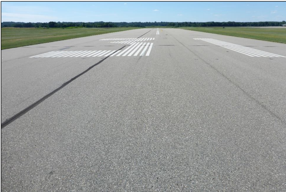
12Y RY1331 001 (PCI = 84) Photo taken pre-maintenance (crack seal and slurry seal)
