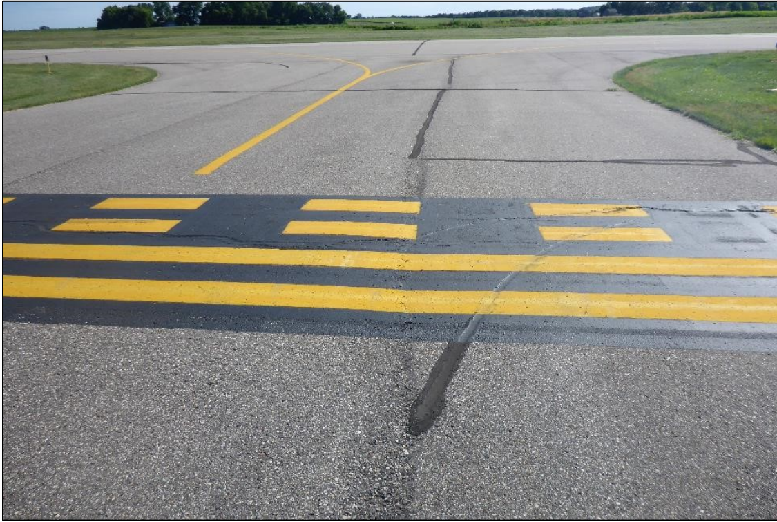
12Y CTA 001 (PCI = 84) Photo taken pre-maintenance (crack seal and slurry seal)
